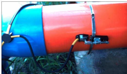
Figure 7. Transducers for ultrasonic flowmeter attached to 10-inch irrigation pipe
