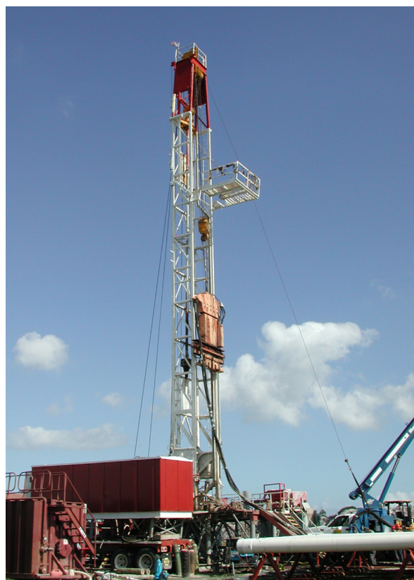
Figure 1. Typical well construction with hollow stem rotary drilling rig. Credits: B. Boman. 2003.
