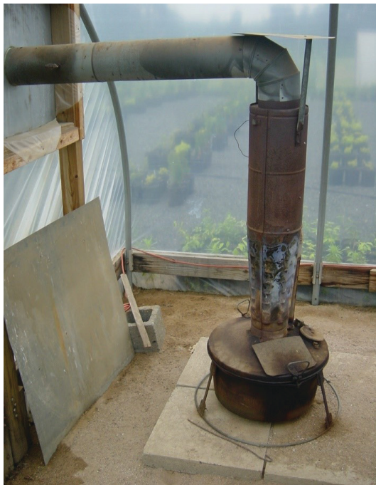
Figure 5. Radiant heaters like these are not recommended for greenhouse heating.
