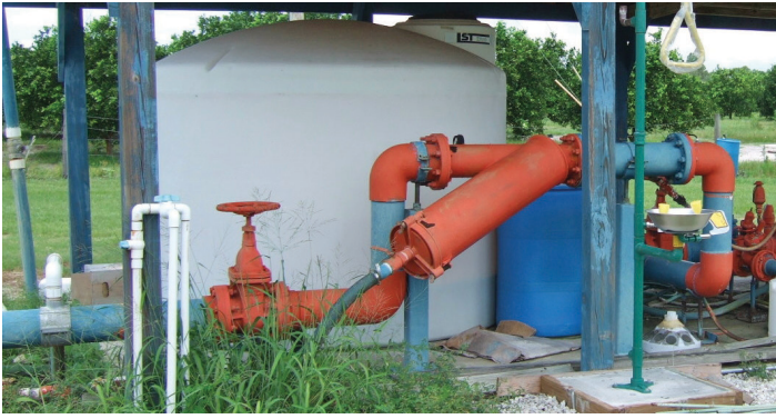
Figure 2. Nutrient solution sources for fertigation are stored in large plastic tanks at the irrigation pump station.
