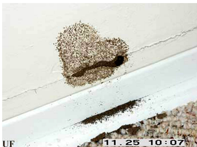
Figure 6. Prorhinotermes simplex (Hagen) termite flight tube emerging from interior wall above molding. Credits: Rudolf H. Scheffrahn, University of Florida
