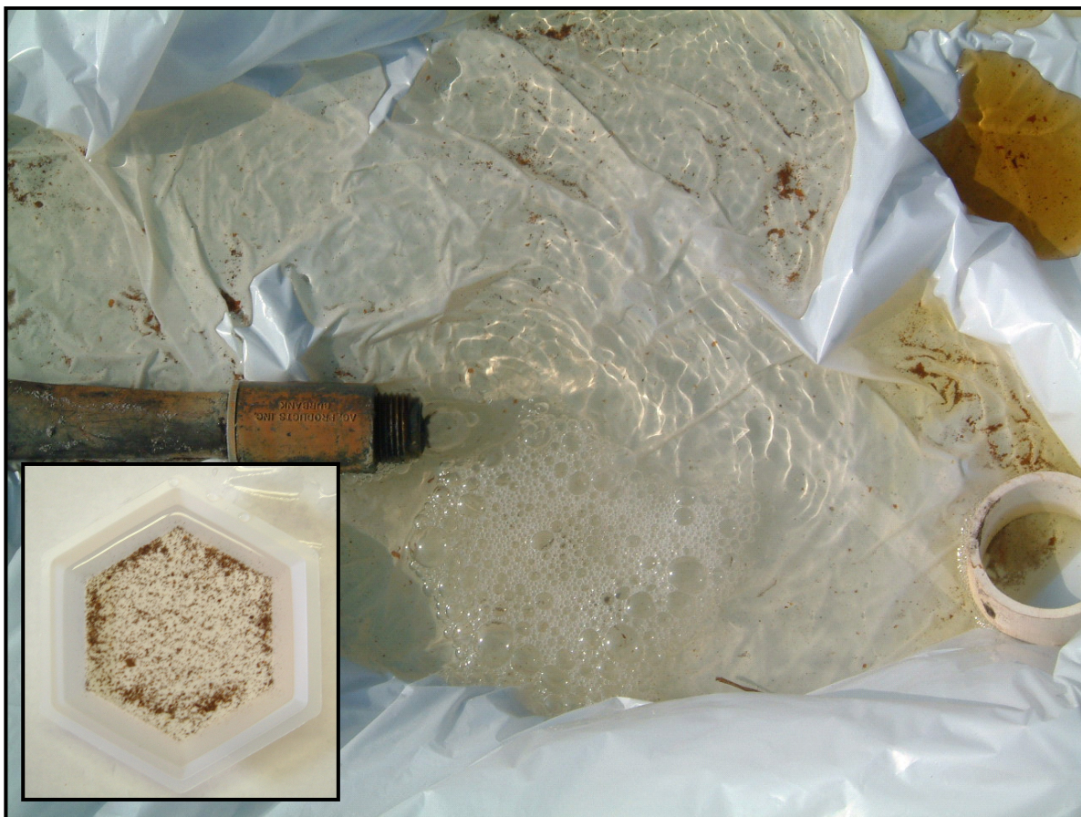
Fig. 1. Catching material flushed from lateral tubing helps estimate the amount of scale in the tube and its composition. In this case, the flushed material appears to be iron-based scale (inset).
