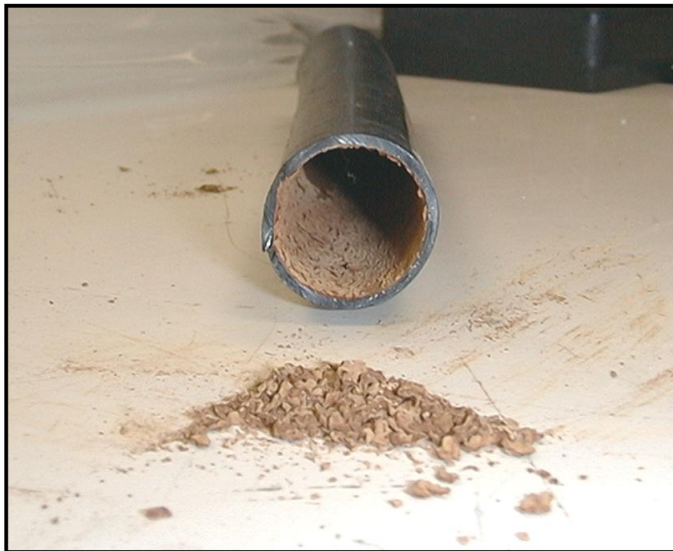
Fig. 7. Severe scaling caused by iron precipitation.
