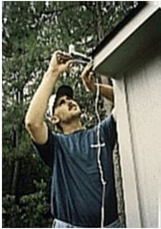
Figure 3. Check to be sure rain sensors are functioning well.
