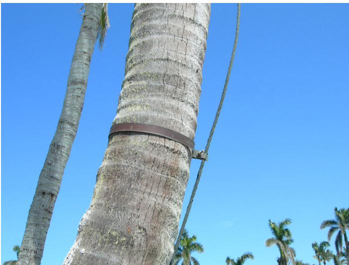
Figure 18. Close-up of the down cable that carries the current to the ground. Credits: A. D. Ali, The Davey Tree Expert Co.
