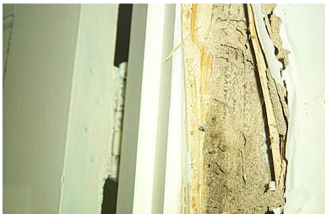
Figure 9. Carton material in door casing damaged by Coptotermes havilandi Holmgren, Key West. Credits: Mark Lang
