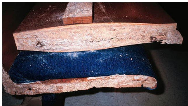
Figure 8. Damage by Coptotermes havilandi Holmgren to church pew, Miami. Credits: B. Maharajh
