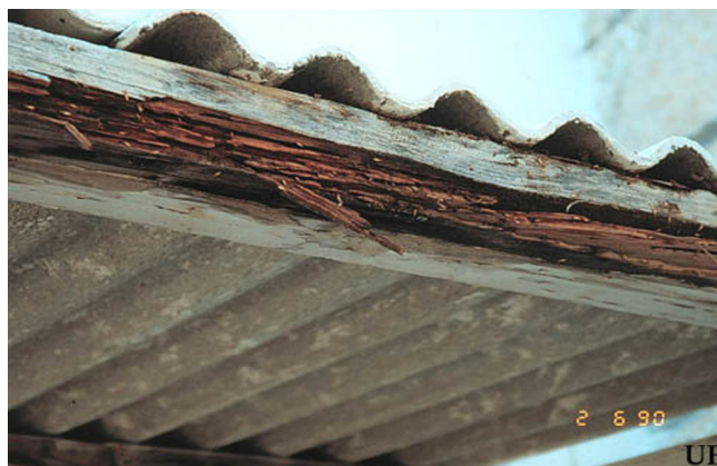
Figure 7. Damage by Coptotermes havilandi Holmgren to fascia, Grand Turk Island. Credits: Rudolf H. Scheffrahn, University of Florida
