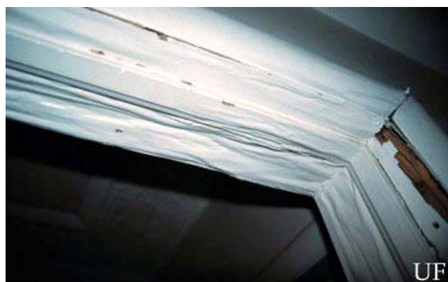
Figure 8. Blistered wood surface damage caused by the Formosan subterranean termite, Coptotermes formosanus Shiraki. Credits: Nan-Yao Su, University of Florida
