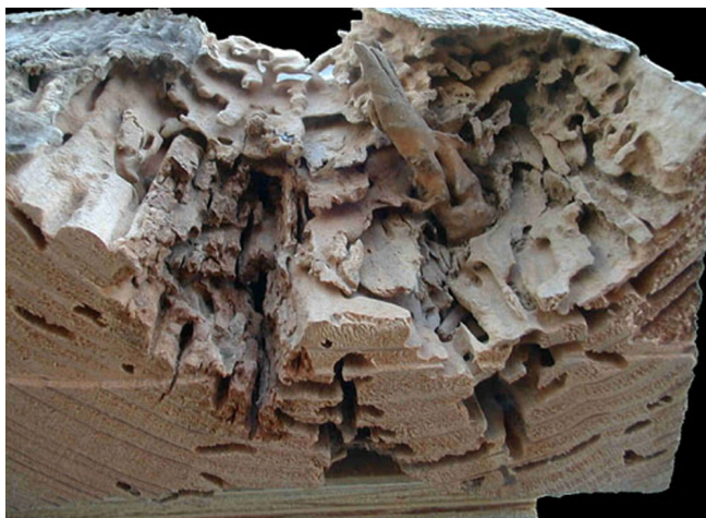
Figure 17. Neotermes jouteli (Banks) damage in 4-inch x 8-inch beam removed from a house in Ft. Lauderdale. Credits: Rudolf H. Scheffrahn, University of Florida
