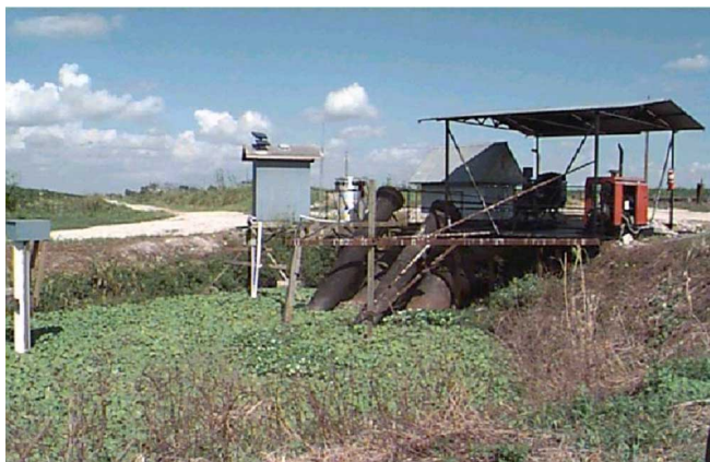
Figure 8. Aquatic weed mats migrated downstream to pump station.
