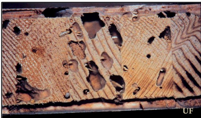
Figure 7. Damage (wooden door) caused by the West Indian powderpost drywood termite, Cryptotermes brevis (Walker). Credits: Rudolf H. Scheffrahn, University of Florida
