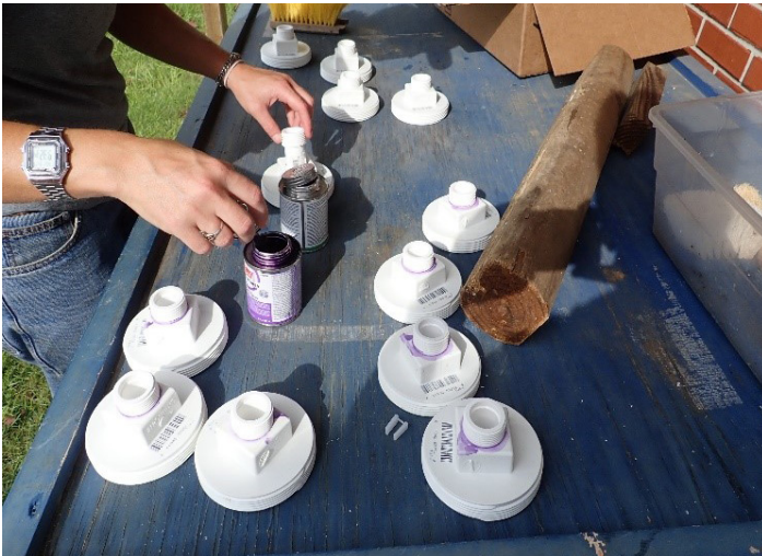
Figure 10. The repair coupling is glued to the threaded cap for the top section of the siphon.
