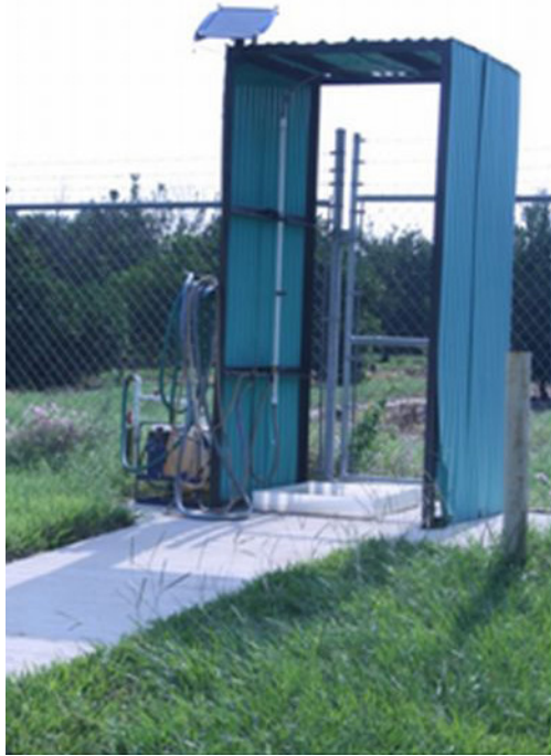
Figure 11a. Automatic personnel decontamination station. Credits: UF/IFAS
