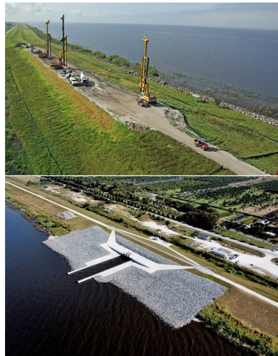
Figure 5. The US Army Corps Herbert Hoover Dike Rehabilitation Project, begun in 2007, includes installation of concrete cut-off walls in the center of the earthen dike (top photo) as well as repair or replacement of the inflow/outflow structures (bottom photo). Credits: US Army Corps of Engineers
