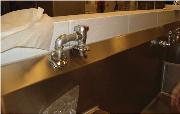
Figure 6. German cockroaches using unsealed escutcheon plates in a cafeteria sink as harborage. Inspection practices should include checking for unsealed openings such as missing or loose pipe and conduit escutcheon plates.
