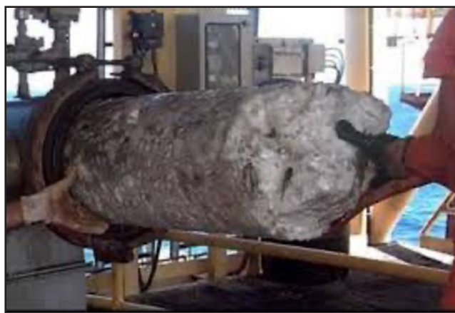
Figure 2. Clathrate-hydrate plug in a gas pipeline. Often, silica particles in the gas stream serve as heterogeneous-nucleation sites [9]
