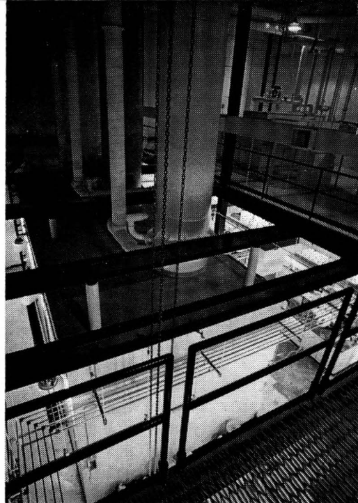
A top view of the high pressure test cells showing the large vertical vent stacks.
