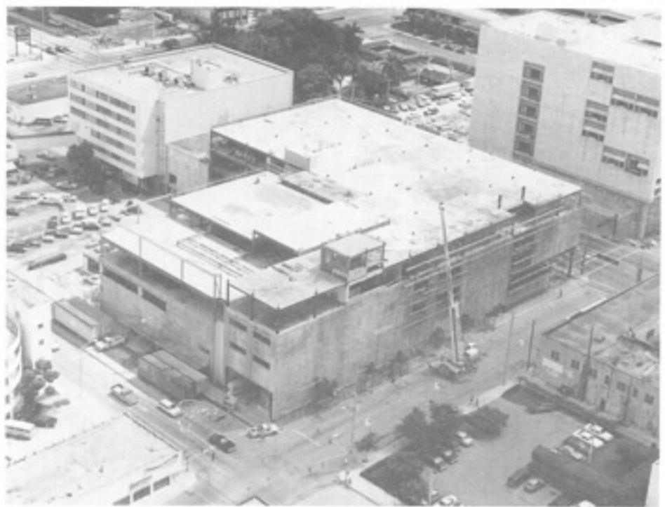
Workmen transform the downtown Burdines store into the Broward County Governmental Center in August 1983. Across Andrews Avenue, in the top right corner of this photo, is the county's main library building, also under construction (photo courtesy of Smith Aerial Photography, Inc.).
