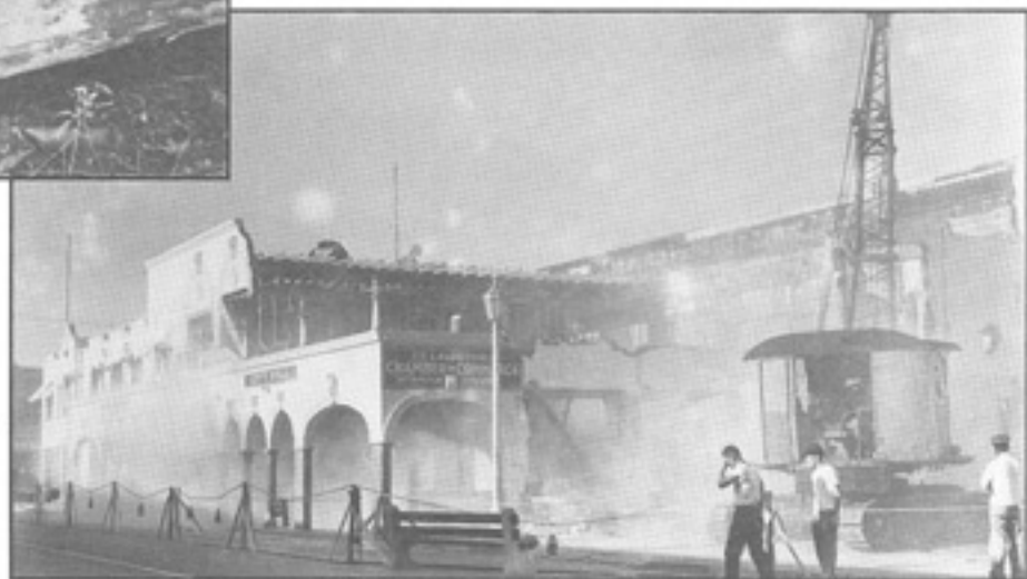
Demolition of the old Fort Lauderdale City Hall at Andrews Avenue and Southwest Second Street, May 1946, to make way for the construction of Burdines department store (now the Broward County Governmental Center).
