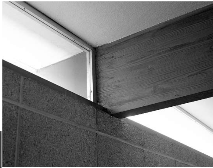
Fig. 8a – Clerestory ribbon windows at Jaffe-Garrett House (built 1959) Provide glimpses of the sky. [photo by Louis Friend, 2006]
