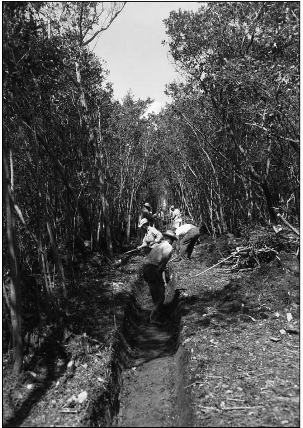
Here workers dig “mosquito ditches” in the central part of Broward County—channels to drain the local marshes where these insects bred—in the mid 1950s. (Image courtesy Fort Lauderdale Historical Society, Gene Hyde Collection)
