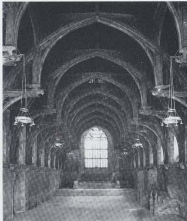
Figure 4. Hammerbeam Roof, Great Hall, Westminster Palace, Courtesy of the Royal Commission on the Historical Monuments of England.
